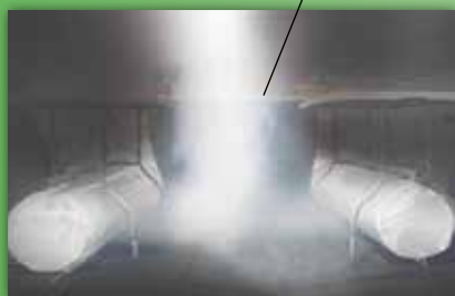
High velocity discharge causes localized drafts.
